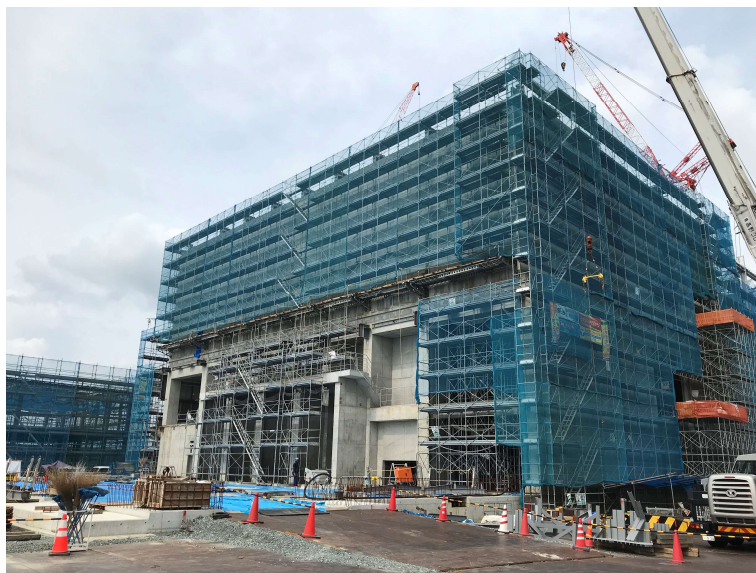
Photo-1 Project of Kikuchi Environmental Preservation Association (commercial operation will start from Mar. 2021)
