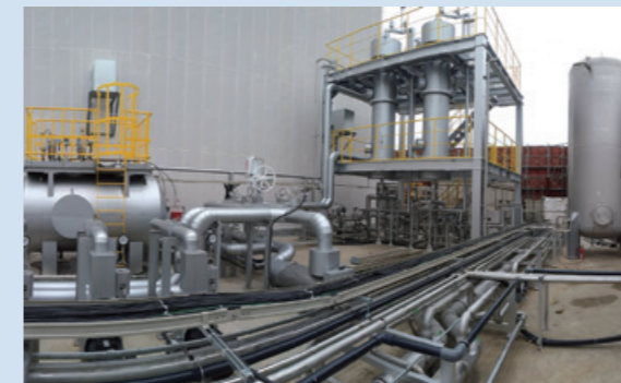
Methanation demonstration facility
