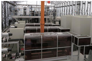
Hydrogen Production Systems
